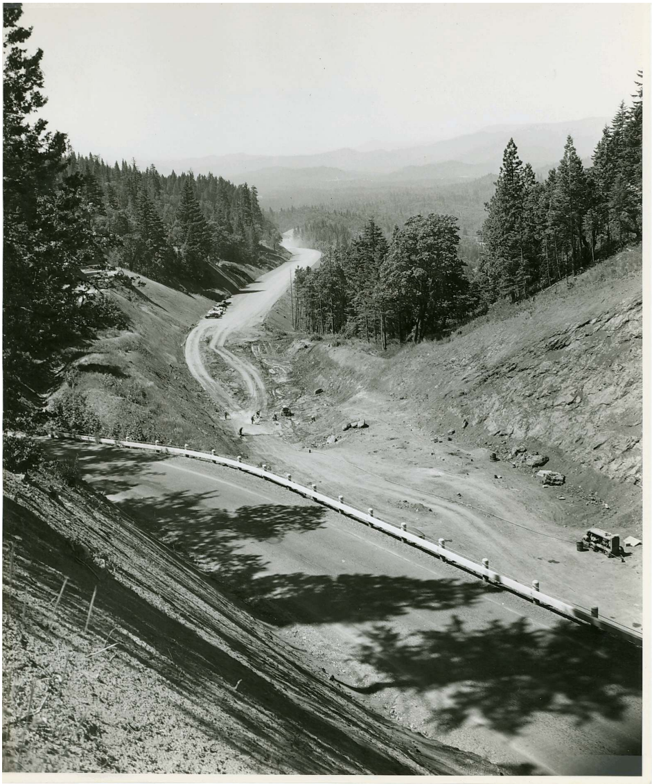
Taking out lower cut thru Summit. Looking S. from S. side of summit cut. Detour in foregrou & finish grade in background. Grave Cr.-Jumpoff Joe Cr. Sec., Pac. Hwy. #1845
