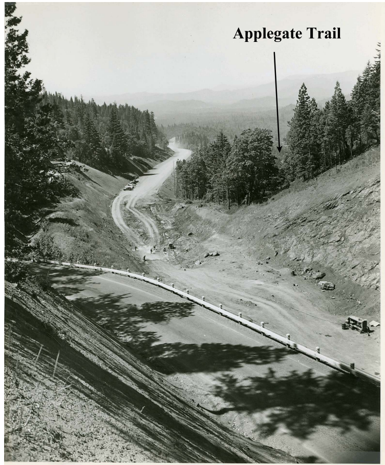
Taking out lower cut thru Summit. Looking S. from S. side of summit cut. Detour in foreground & finish grade in background. Grave Cr.-Jumpoff Joe Cr. Sec., Pac. Hwy. #1845
