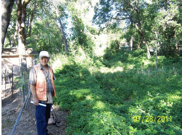
Photo 4. Kelly Rarey on Dike Protecting School From Winter Flooding of Vannoy Creek
