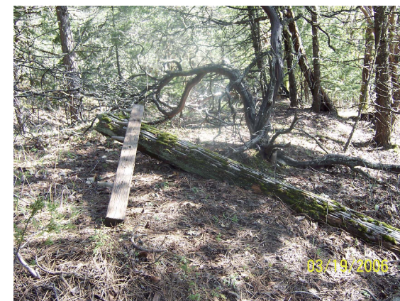
AT & T Long Distance Telephone Line Parts: Cross Arm & Pole At Sexton Mt.
