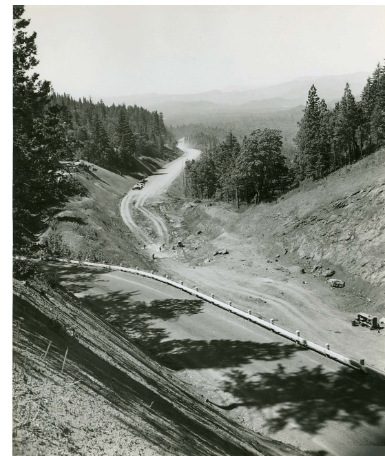
Taking out lower cut thru Summit. Looking S. from S. side of summit cut. Detour in foreground & finish grade in background. Grave Cr.-Jumpoff Joe Cr. Sec., Pac. Hwy. #1845
